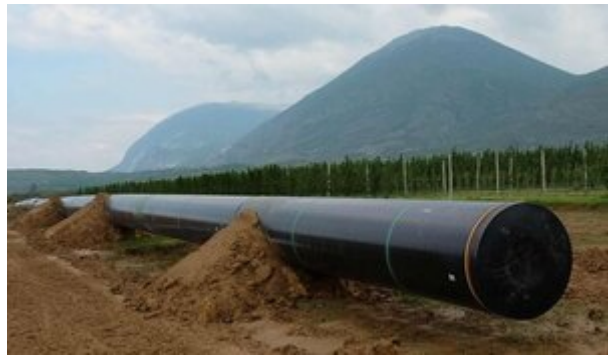
Southern Gas Pipeline © Ido Iiven
