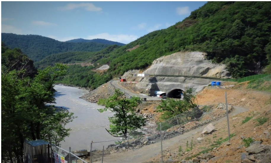
Lower Namakhvani dam and tunnel construction site, July 2021. Credit: Andrey Raley, CEE Bankwatch Network
