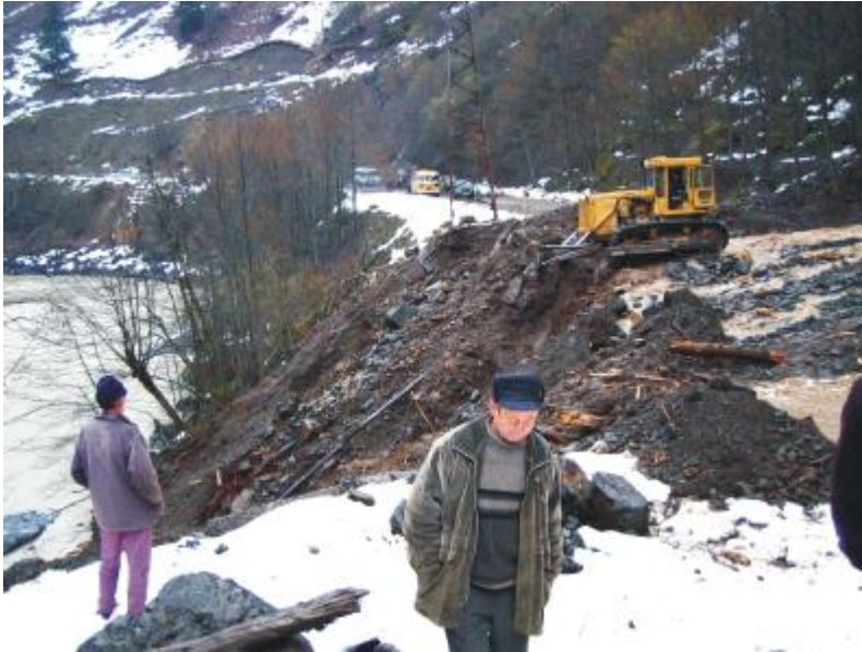
The landslide on the Khudoni site
