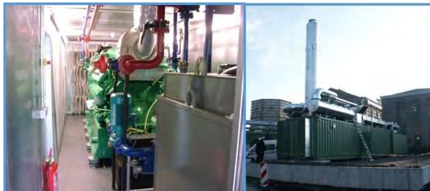
Figure 19 Compact Mobile Power Plant
