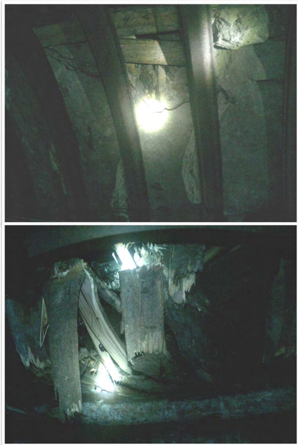
Figure 21 Damaged Roadways at Mindeli Mine
